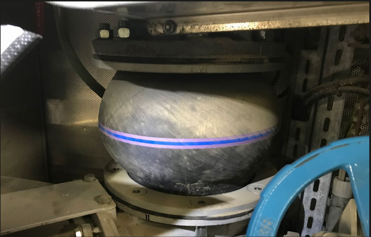
FPM rubber joint \varnothing 300 mm for 1 bar operating pressure and 180° C, installed on an ash chute
