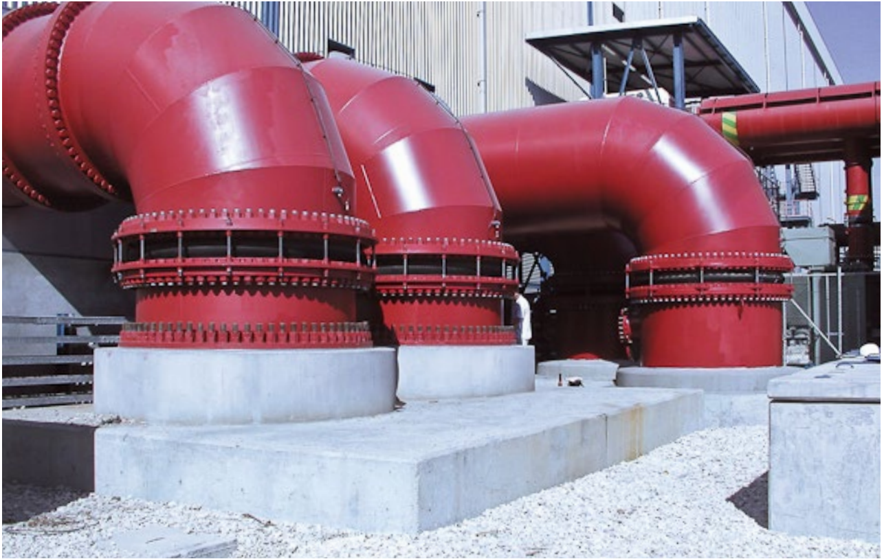
Sea water intake cooling water line \varnothing 2,600 mm, operating pressure 2.5 bar, lateral tied rubber expansion joints of type U111M
