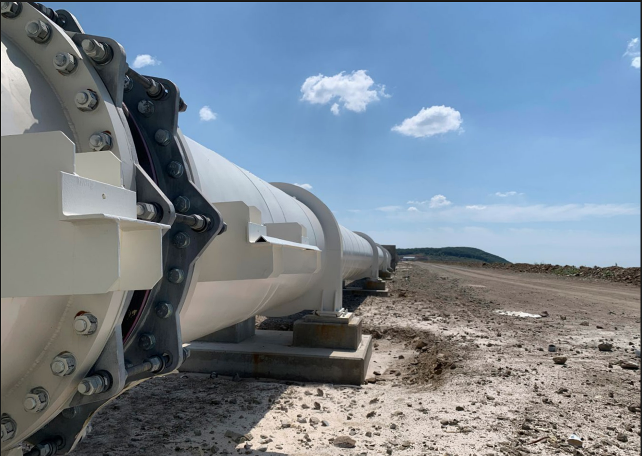
Installation of tied rubber expansion joints \varnothing 1,400 mm in a ring water line of a copper mine
